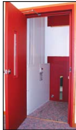
Fired rated steel door
